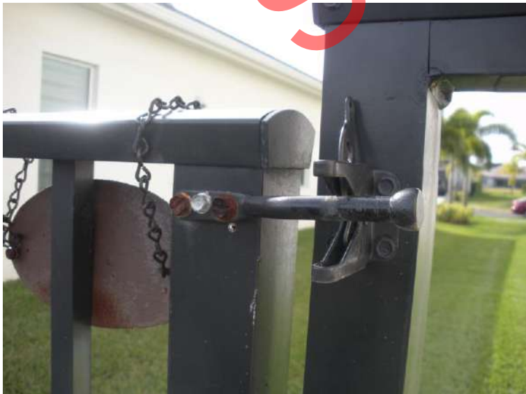
Gate is not operable as per standards. Adjustment is recommended.
