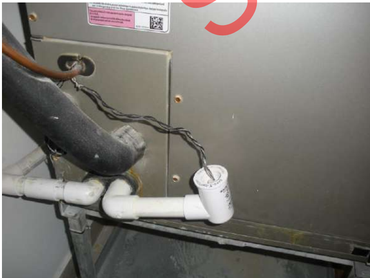
Flow switch is not on the standard position. Elevated flow switch position prevents the proper functionality of the float to shut off the unit in time of need.
