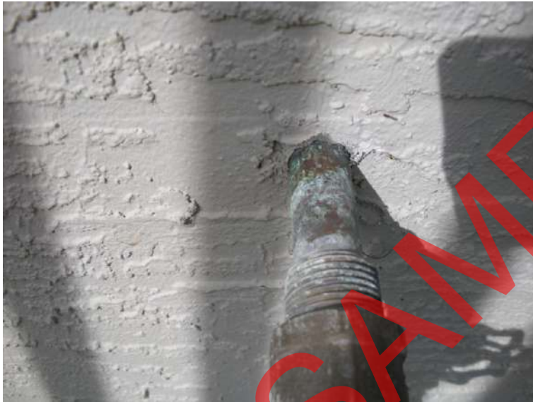
Pipe is not watertight, siliconing is recommended to prevent water intrusion.
