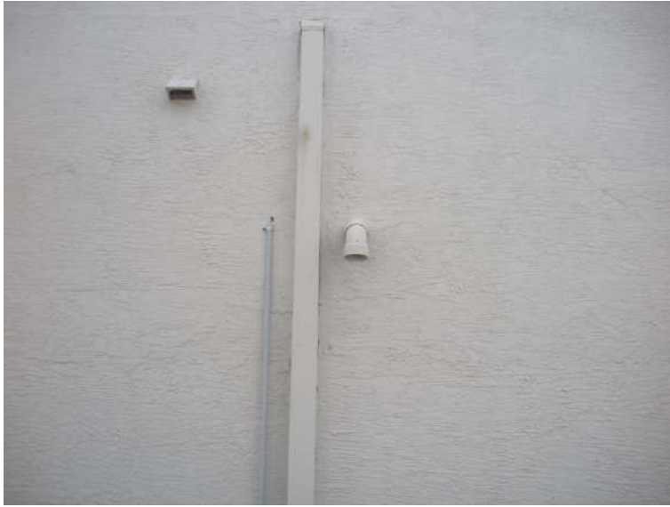
Gas water heater ducting pipe
