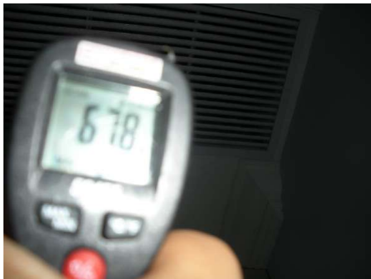
HVAC temperature read
