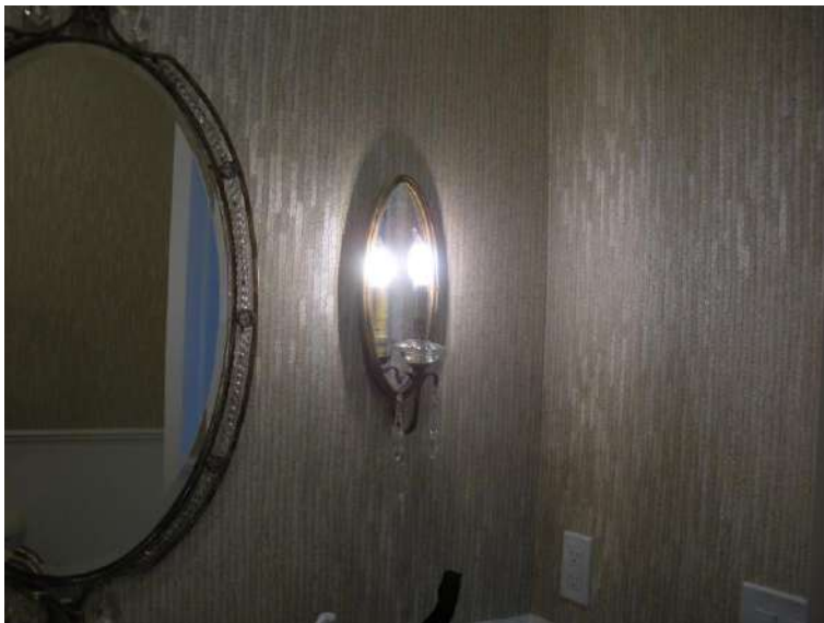
Light fixture is missing globe.
