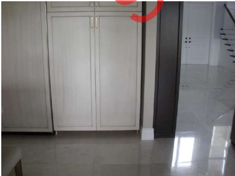
Toe kicks and filler strip are missing in the kitchen cabinetry.
