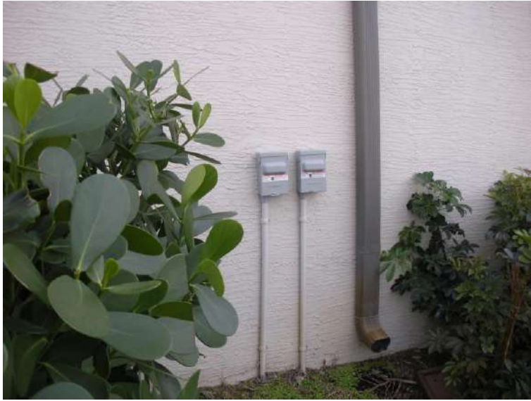
HVAC pull out switches.
