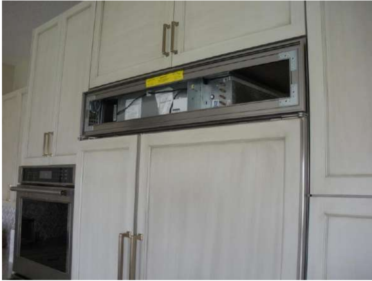
Kitchen shows missing matching panel on the refrigerator.
