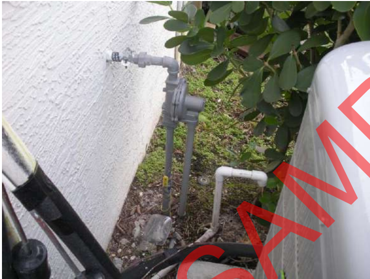
Gas Supply and valve located on the side of the house.
