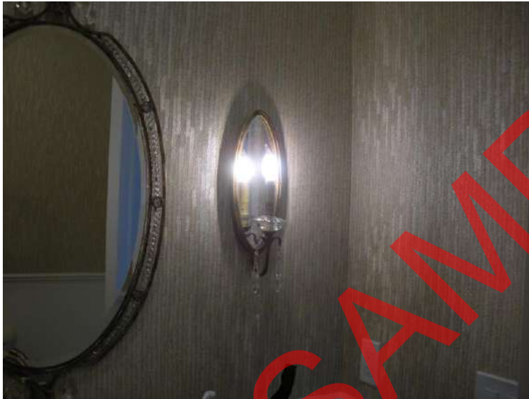
Multiple rooms light fixtures are missing globes.
