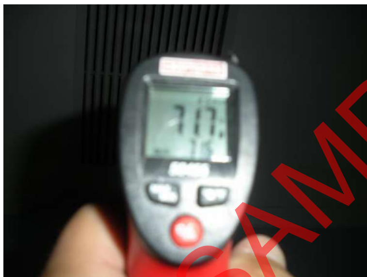
HVAC temperature read
