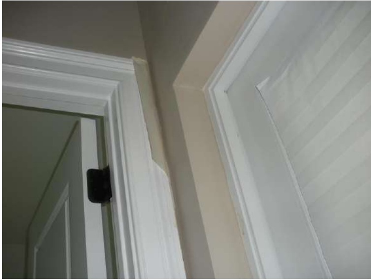
Making tape left behind after painting job.
