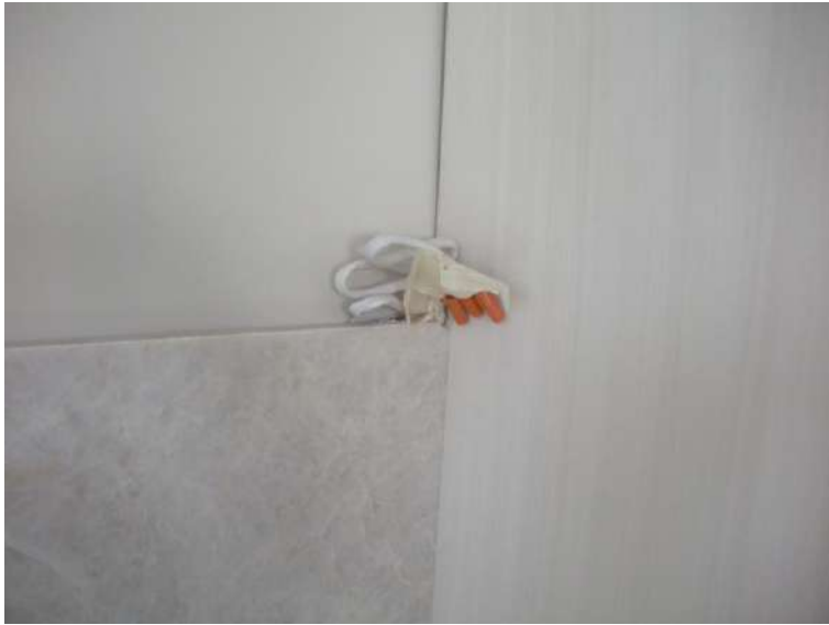
Exposed capped wiring in the kitchen.
