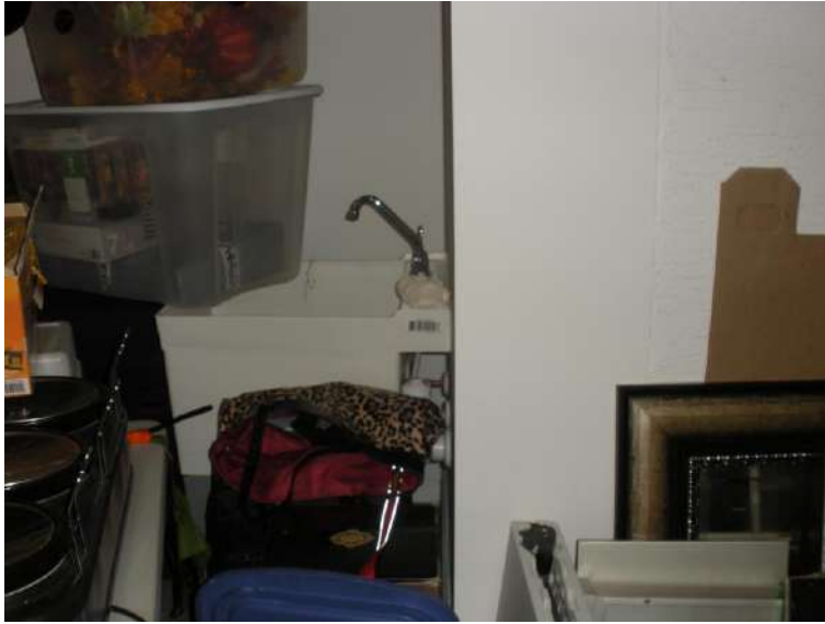
Obstructed sink. No access to inspect.
