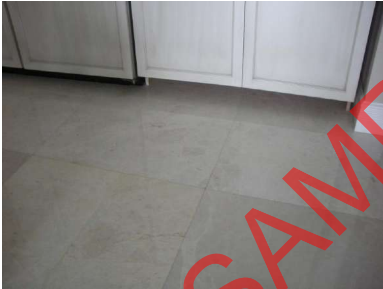
Some toe kicks are missing in the kitchen cabinetry.
