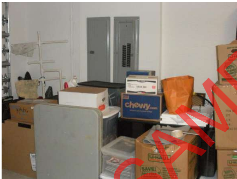
Panels branch circuits were not accessible due to being blocked by personal belongings.
