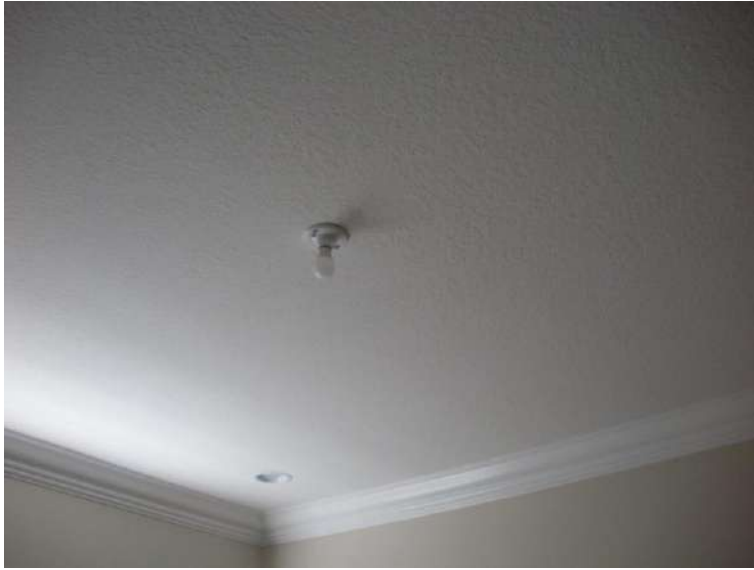
Multiple rooms light fixtures are missing globes.
