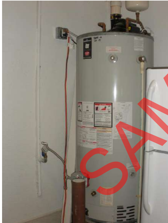
Gas Water Heater
