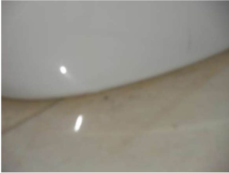
Toilet missing grout at the base.
