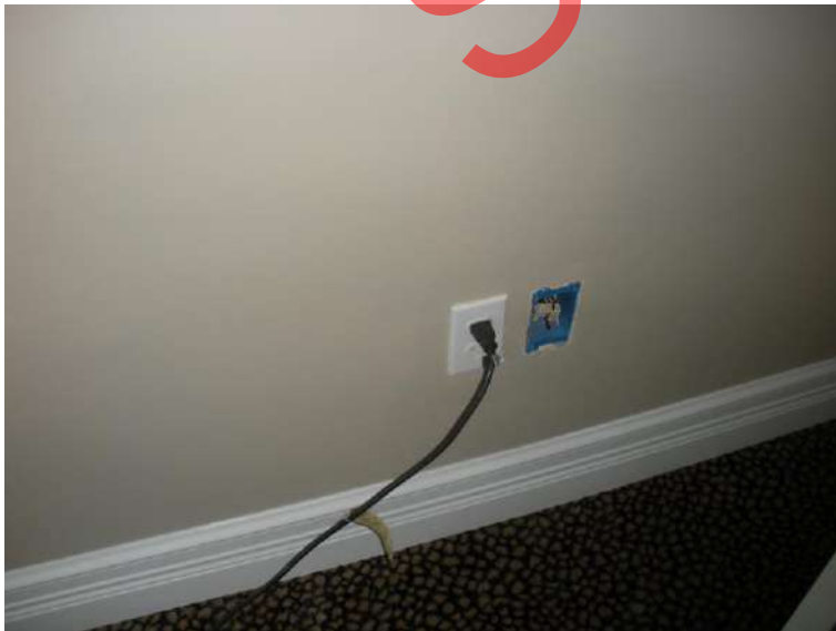
Exposed wiring in box. Cover plate installation is recommended.
