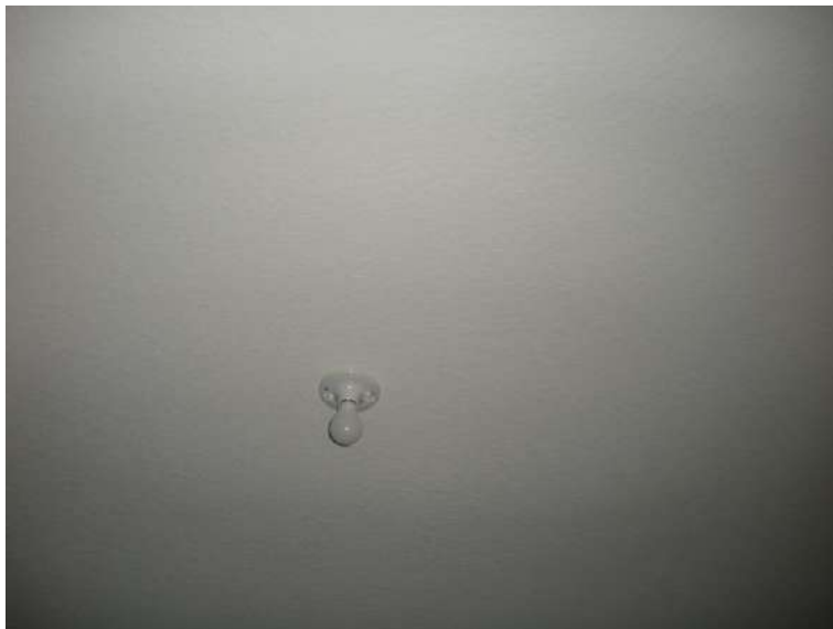
Multiple rooms light fixtures are missing globes.
